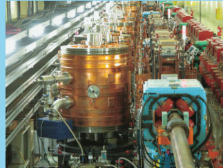
RF cavity with a large energy storage cavity
