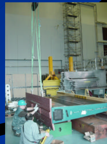
A special module for which the connecting plate is a single piece has a key which sits in the slots shown in the saddle. The key carries the vertical shear load in the cylinder which is transferred through the saddle to the ATLAS support rails..
