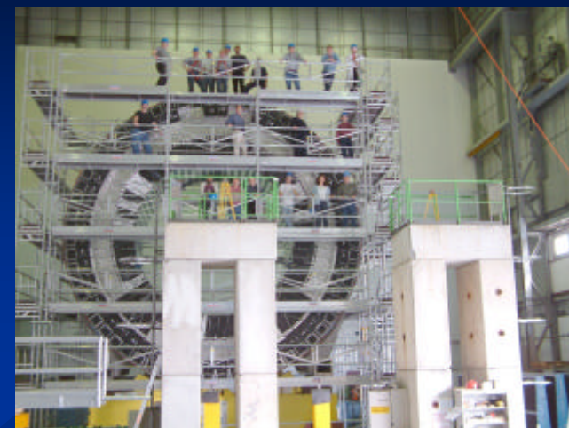
A full pre-assembly of each cylinder will be carried out prior to final assembly in the ATLAS cavern. The first of these is shown here. The assembled cylinder is itself over 8m high, weighs 640 tons and sits on 2 pairs of blocks below each of the saddle beams.
